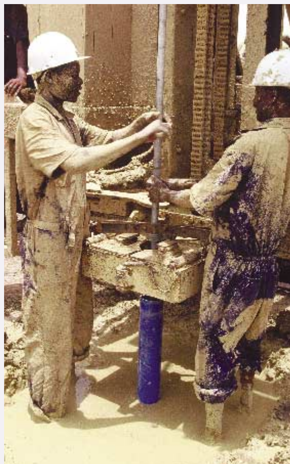
Drilling of water well sponsored by Lundin Sudan Limited along the all weather road between Rubkoena and Thar Jath (Block 5A in Sudan)
